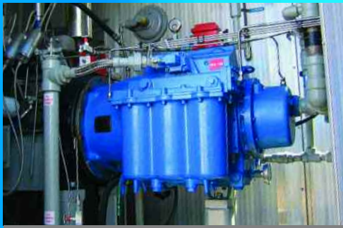
Well head pumping
